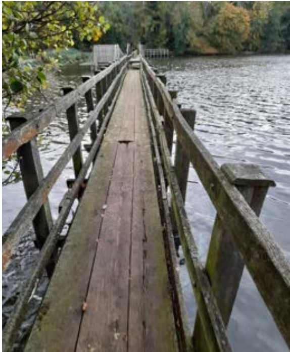
Unsafe rotting bridge
